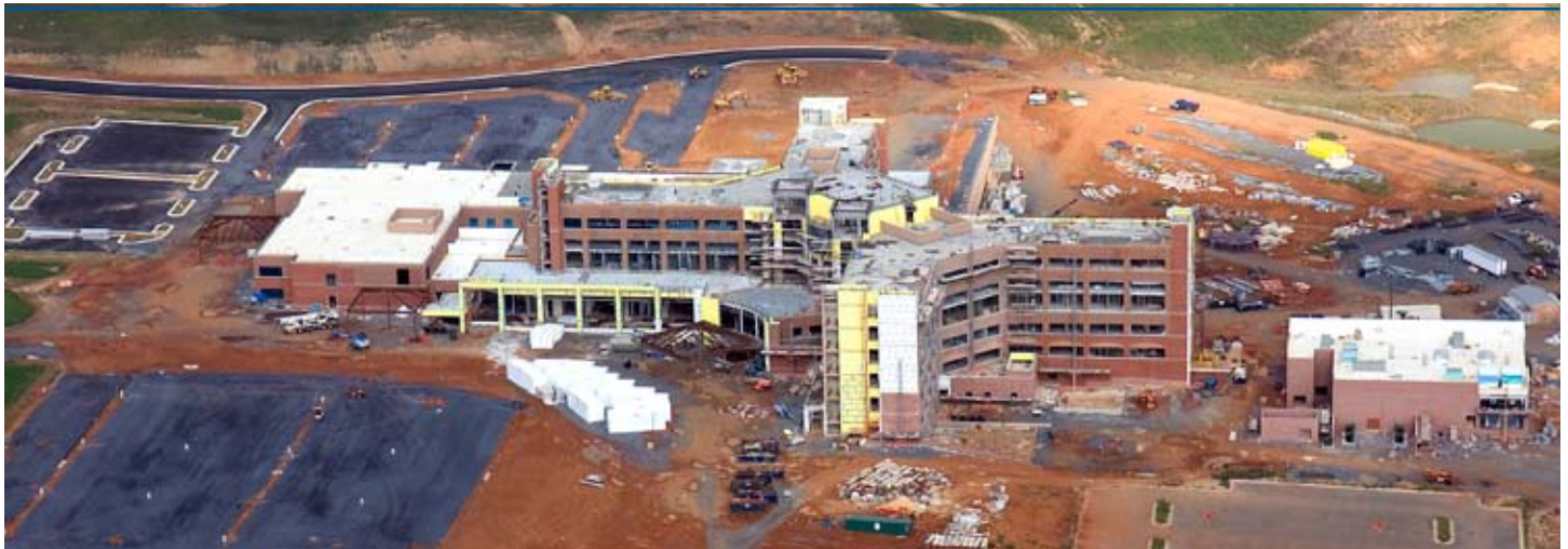
Construction is moving quickly on the new hospital, as seen in this aerial view of the front entrance to the building. Photo by Tommy Thompson.
