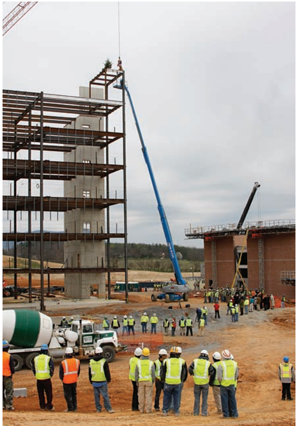
Bovis Lend Lease and RMH team members look on as the last steel beam is placed on the new hospital structure at a "topping out" ceremony April 3. Hundreds of RMH employees, volunteers and physicians signed the beam.
